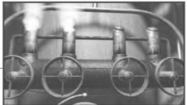
Fig. 3-43. Final setting for the middle tier—two open valves venting hot air.
