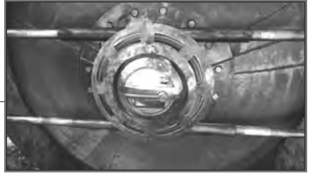
Fig. 3-15. The gear platform door can open once power lights up the lock mechanism.
