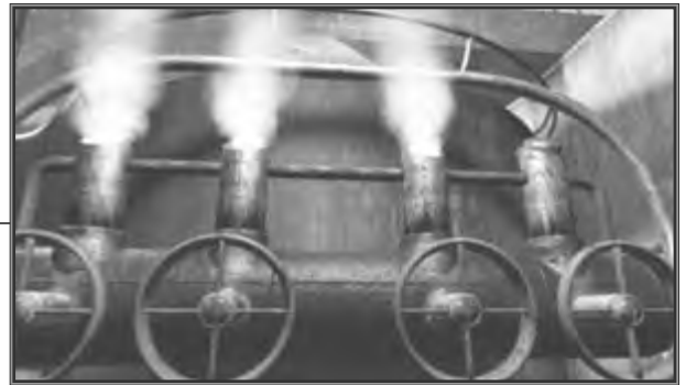
Fig. 3-42. Final setting for the top tier—three open valves venting hot air.
