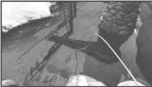
Fig. 3-4. This power cable runs from the stone structure down into the water.
