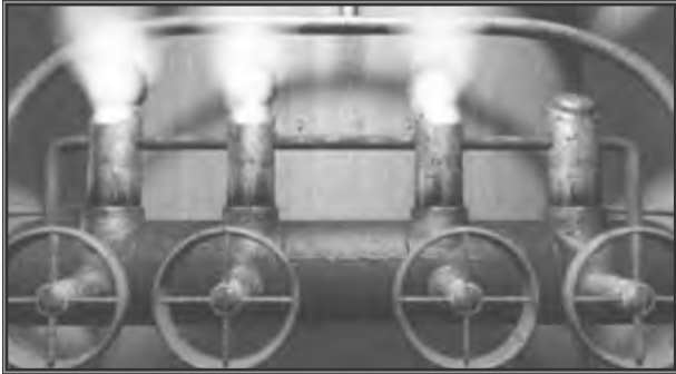
Fig. 3-44. Final setting for the bottom tier—three open valves venting hot air. (The jammed valve stays closed.)
